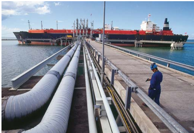
An LNG ship docked at Point Fortin in T&T where future gas production looms large. Photograph by Barry Lewis.
