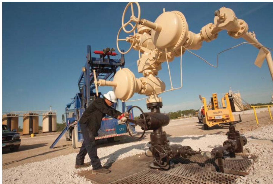
A Swift Energy Co. field technician uses a slick line unit to finish a pressure gauge run in the AWP field in south Texas. Swift is exploiting the Eagle Ford shale formation in the field for oil. See article on Eagle Ford shale play on Page 4.
