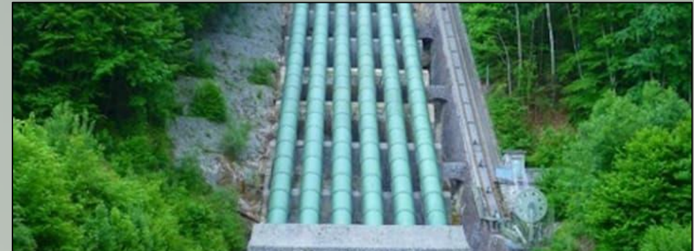
Onshore Transmission Lines
