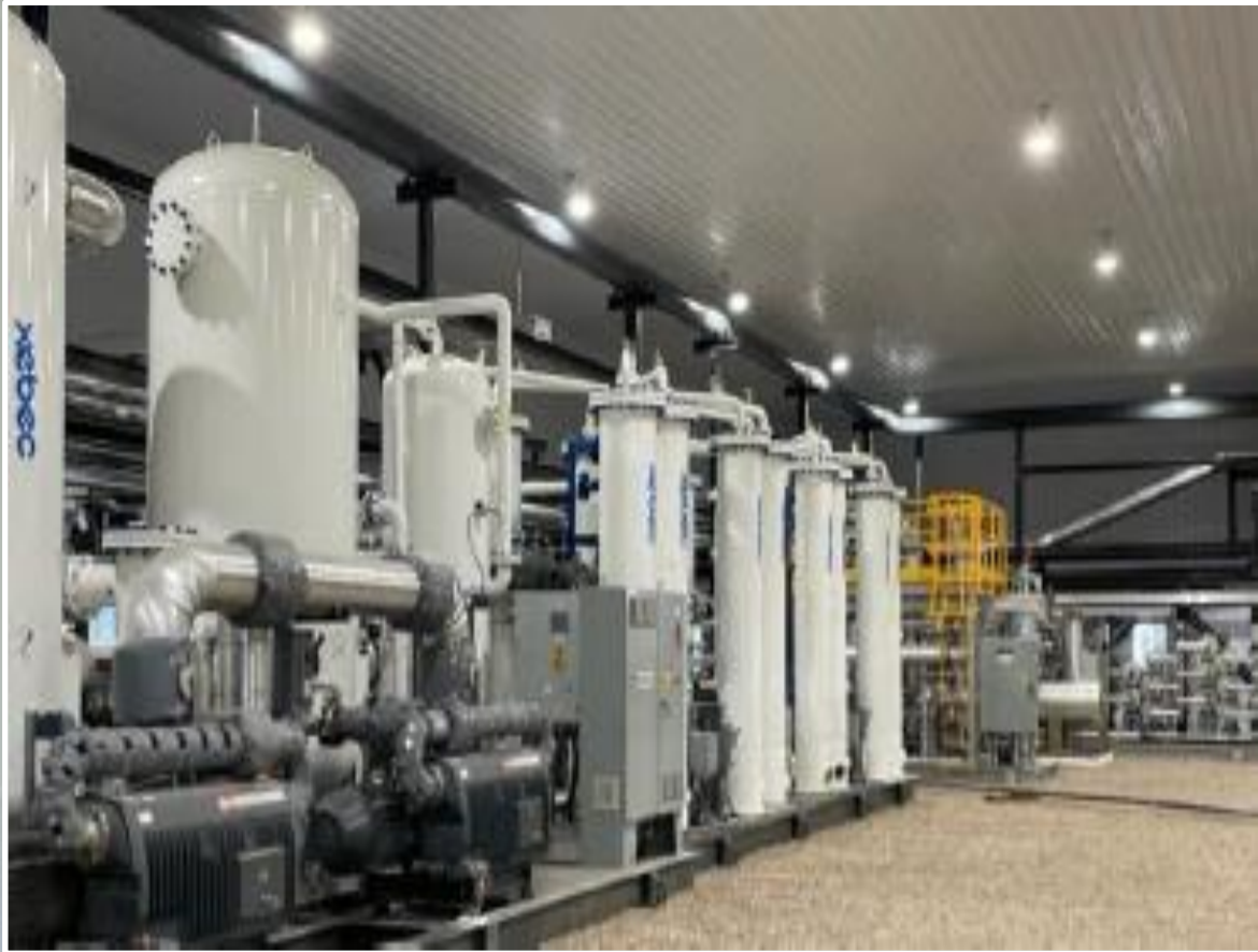
Helium Purification Facility
